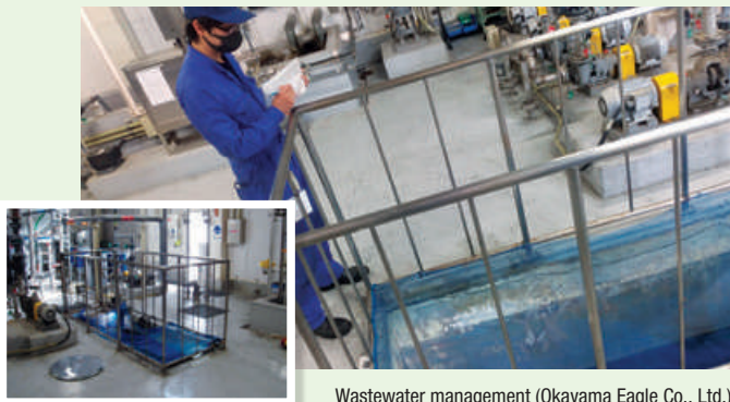
Wastewater management (Okayama Eagle Co., Ltd.)
